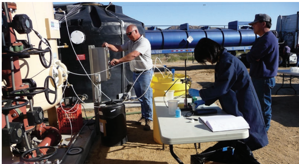
EPA contract workers perform testing on TPWD's arsenic removal system. The EPA has partnered with the district to find innovations in arsenic removal that can be shared with districts throughout the nation.
