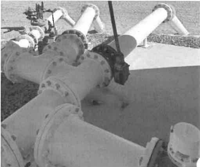
Piping from the existing TPWD Booster Station
