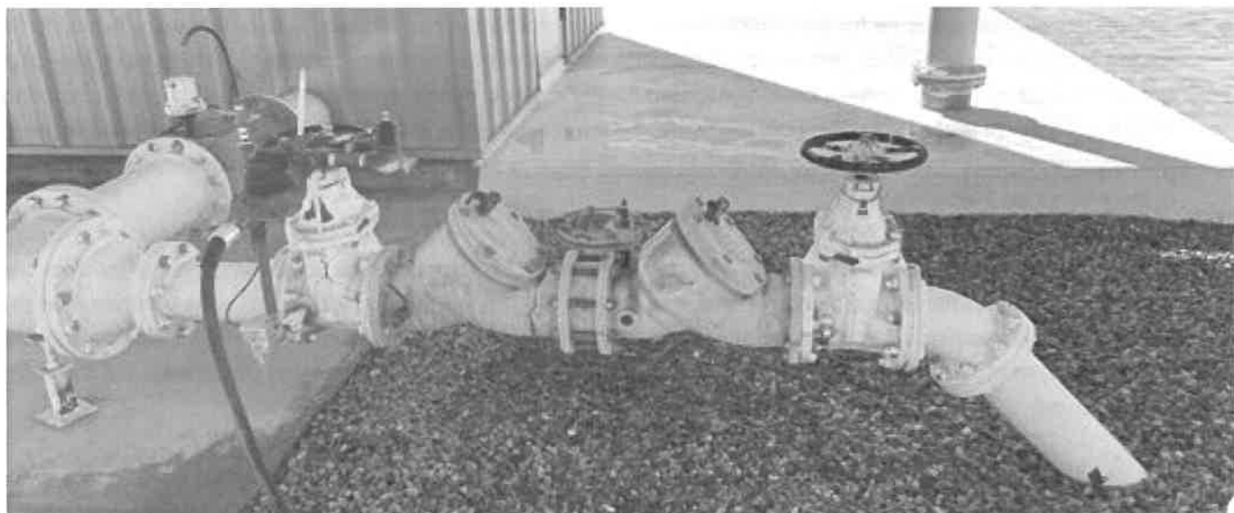
Piping from the existing TPWD Booster Station
