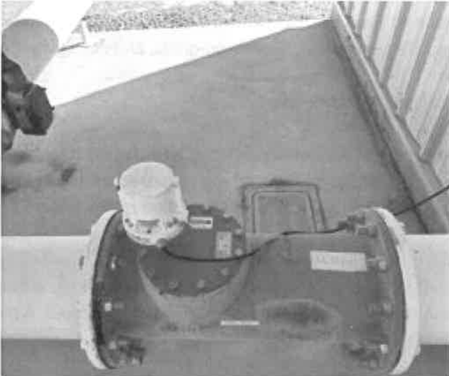
Piping from the existing TPWD Booster Station
